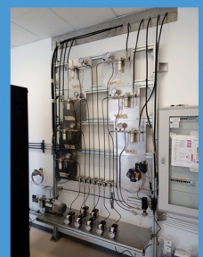
View of the sampling lines
